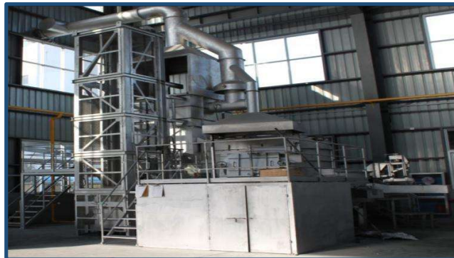
溶錬炉 Central Melting Furnace
